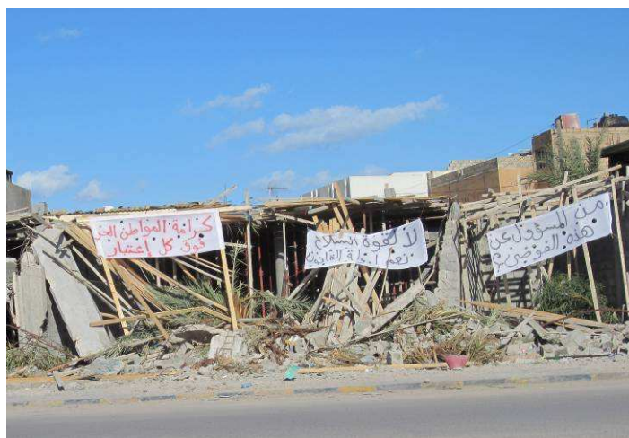
Banners put up by a man on his house, which had been demolished by militias in Misratah. From left to right they read: "Dignity of free citizens comes first", "No to the power of weaponry and yes to a country of law", "Who is responsible for this chaos?" February 2012 © Amnesty International
